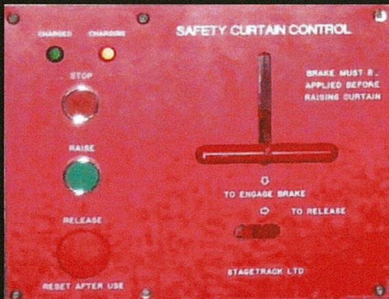
Main Control Panel/ Manual Release
